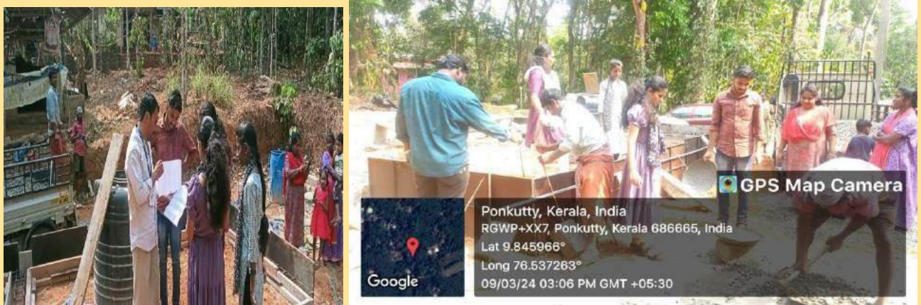
Figure 2: NSS Volunteers involved in the activity of filling of concrete in the foundation
